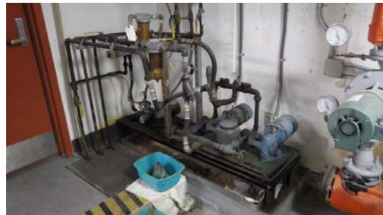
4. HOSPITAL OIL PUMPS
