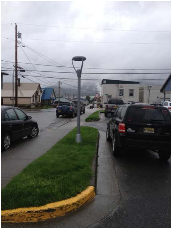
Photo 5: Exterior Light Pole Standard
