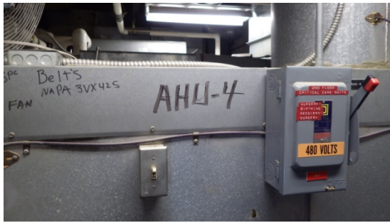
19. HOSPITAL FAN ROOM AHU-4 AIR HANDLING UNIT
