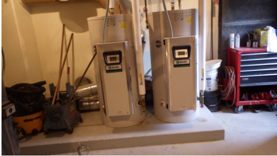
13. LONG TERM CARE FACILITY ELECTRIC HOT WATER TANKS
