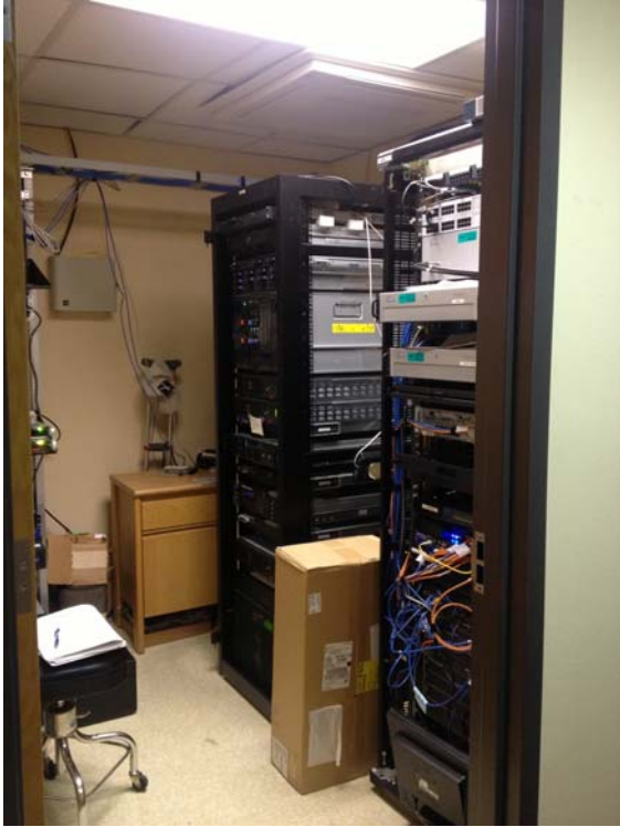
Photo 8: Data Network Equipment
