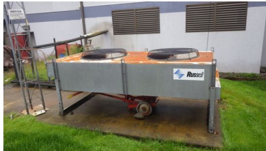
10. HOSPITAL CHILLER EXTERIOR CONDENSERS
