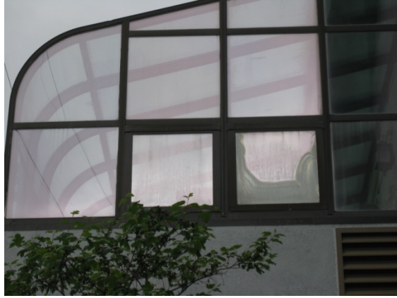
A6 Window Failed Seals
