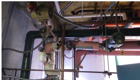
12. HOSPITAL DOMESTIC HOT WATER RECIRCULATION PUMPS
