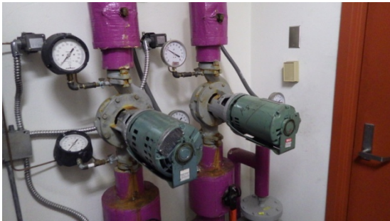
9. HOSPITAL CHILLED WATER PUMPS
