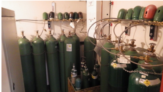
41. HOSPITAL MEDICAL GAS ROOM
