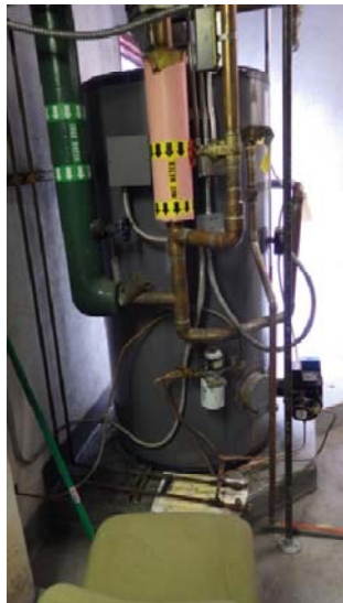
11. HOSPITAL OIL FIRED HOT WATER HEATER
