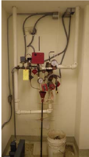
43. HOSPITAL SATELLITE DRY SPRINKLER HEADER
