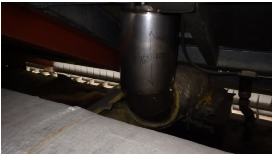
29. LONG TERM CARE FACILITY ATTIC KITCHEN GREASE EXHAUST DUCT
