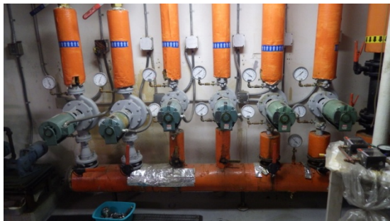
5. HOSPITAL HEATING PUMPS
