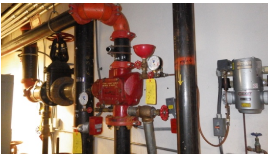
45. HOSPITAL SPRINKLER HEADER
