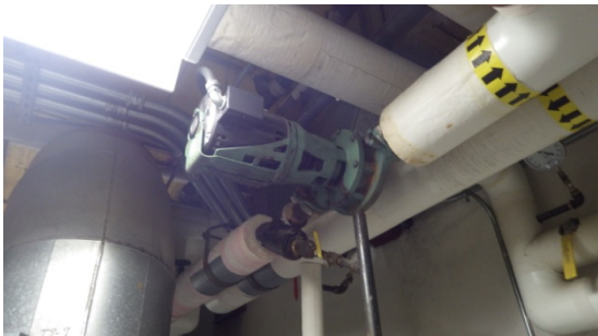
17. HOSPITAL FAN ROOM HEAT RECOVERY PUMP
