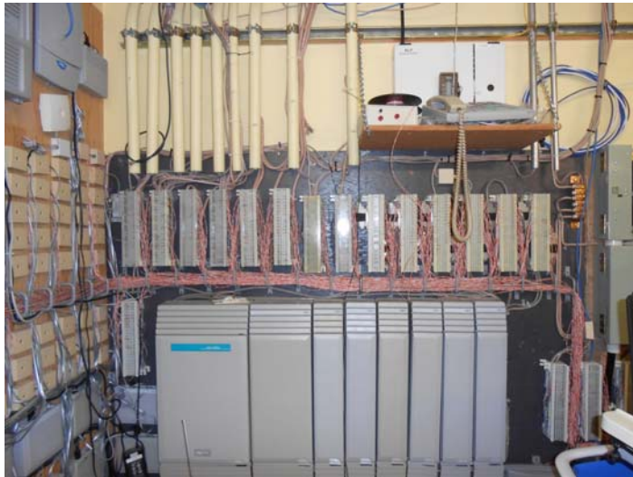
Photo 7: Telephone Switch and System Interconnections
