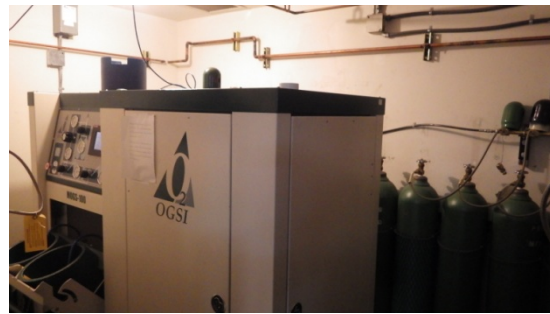
40. HOSPITAL MEDICAL GAS ROOM MEDICAL AIR COMPRESSOR
