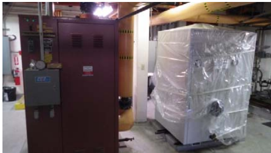
3. HOSPITAL ELECTRIC BOILERS
