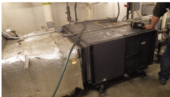
23. LONG TERM CARE FACILITY ATTIC AHU-5
