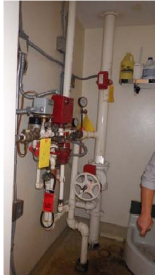
44. HOSPITAL SATELLITE DRY SPRINKLER HEADER
