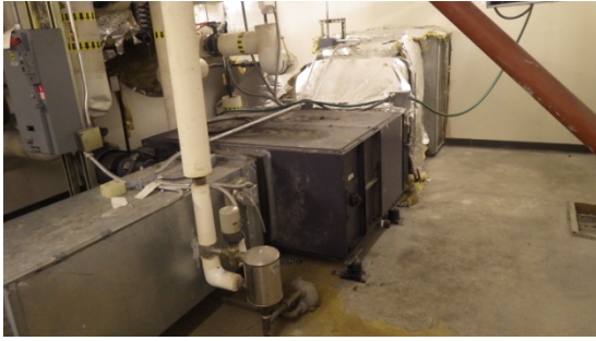
25. LONG TERM CARE FACILITY ATTIC AHU-6
