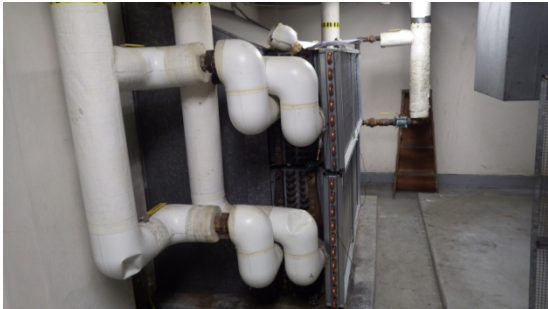
15. HOSPITAL FAN ROOM INTAKE PLENUM WITH HEAT RECOVERY COIL
