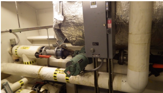
33. HOSPITAL ATTIC RETURN FAN RF-3
