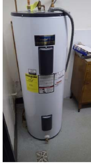
14. HOSPITAL KITCHEN HOT WATER TANK
