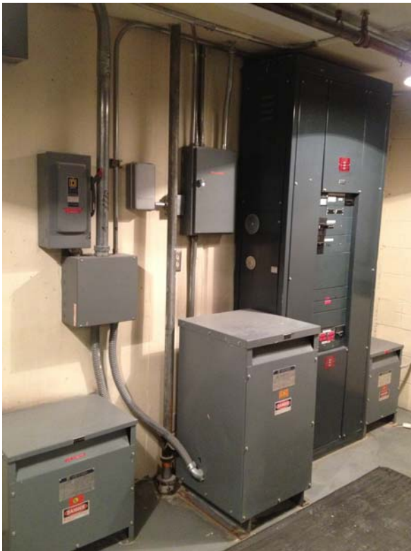
Photo 3: Typical Distribution Equipment
