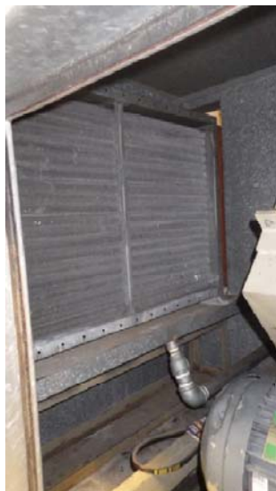
21. HOSPITAL FAN ROOM AIR HANDLING UNIT AHU-4 HEATING COIL
