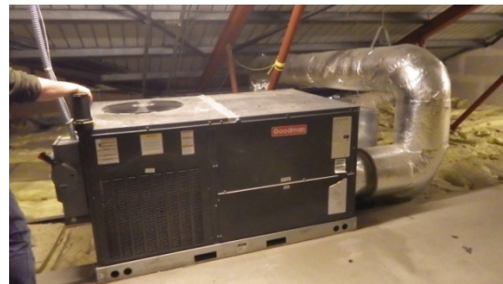
30. HOSPITAL LAB CT ROOM HEAT PUMP AIR-CONDITIONING RECIRCULATION FAN
