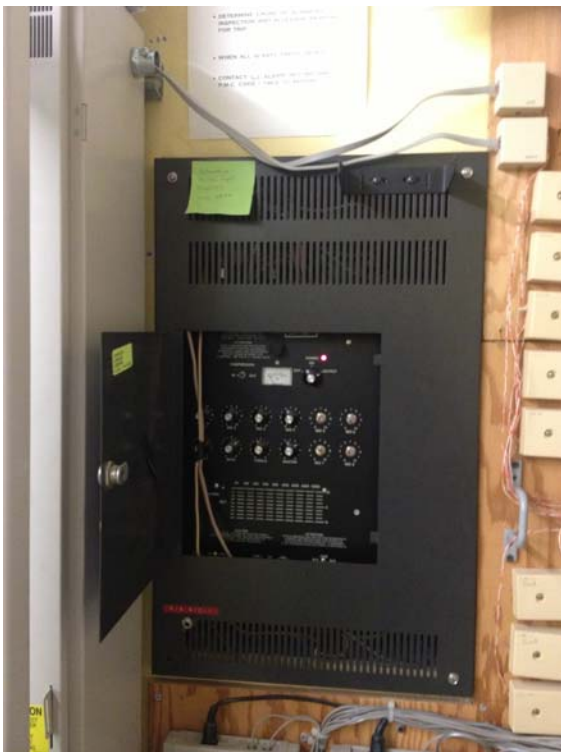
Photo 9: Intercom System Amplifier
