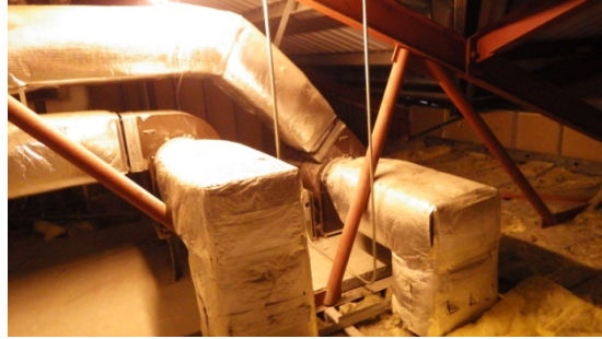
32. HOSPITAL ATTIC TYPICAL EXHAUST FAN
