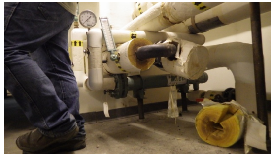
34. HOSPITAL ATTIC RETURN FAN RF-2
