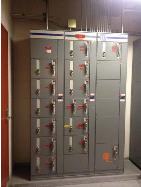
Photo 2: Motor Control Center
