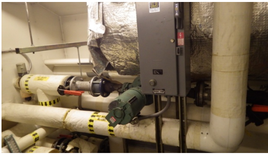
27. LONG TERM CARE FACILITY ATTIC AHU-5 & 6 HEAT RECOVERY PUMP
