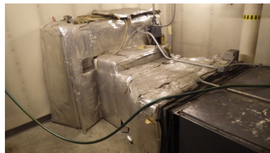
24. LONG TERM CARE FACILITY ATTIC AHU-5 INTAKE PLENUM
