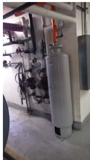
6. MEDICAL CLINIC HEATING PUMPS
