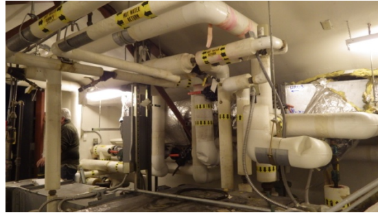
26. LONG TERM CARE FACILITY ATTIC AHU-6 PIPING
