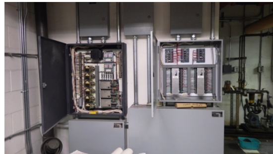
36. HOSPITAL BOILER ROOM MIX OF ELECTRONIC AND DDC CONTROLS
