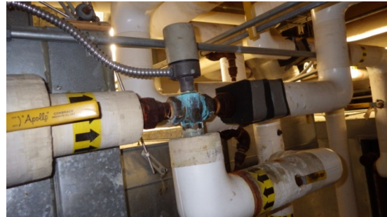
16. HOSPITAL FAN ROOM HEAT RECOVERY PIPING, AHU BEYOND
