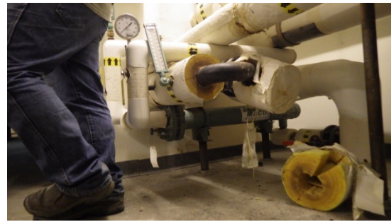
28. LONG TERM CARE FACILITY ATTIC AHU-5 & 6 HEAT EXCHANGER
