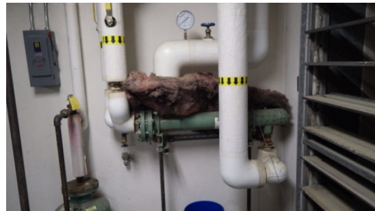
18. HOSPITAL FAN ROOM HEAT RECOVERY HEAT EXCHANGER
