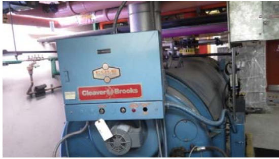
1. HOSPITAL OIL FIRED BOILER
