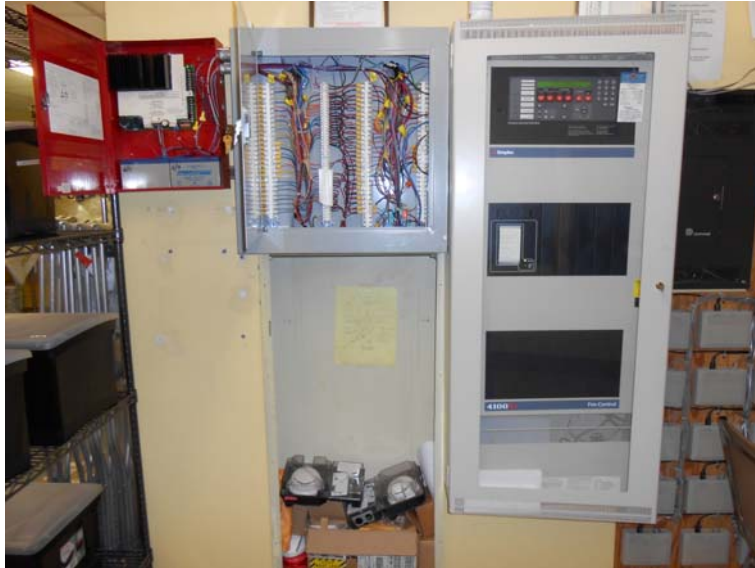
Photo 6: Fire Alarm Control Panel and Accessories
