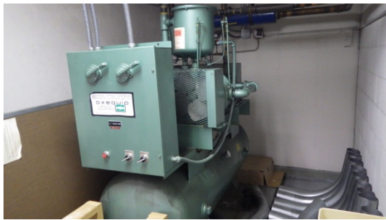
39. HOSPITAL BOILER ROOM VACUUM PUMP
