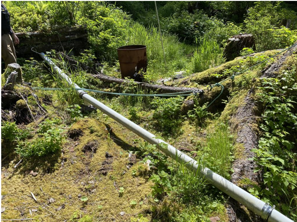
Pipe connected to septic tank.
